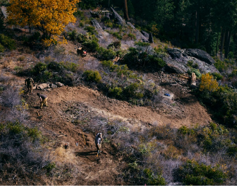
Trail construction on Mt. Hough. Photography: Ken Etzel, Sierra Buttes Trail Stewardship.
