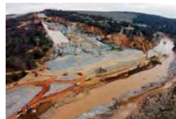
Riverbanks collapse after Oroville Dam spillway shut off
